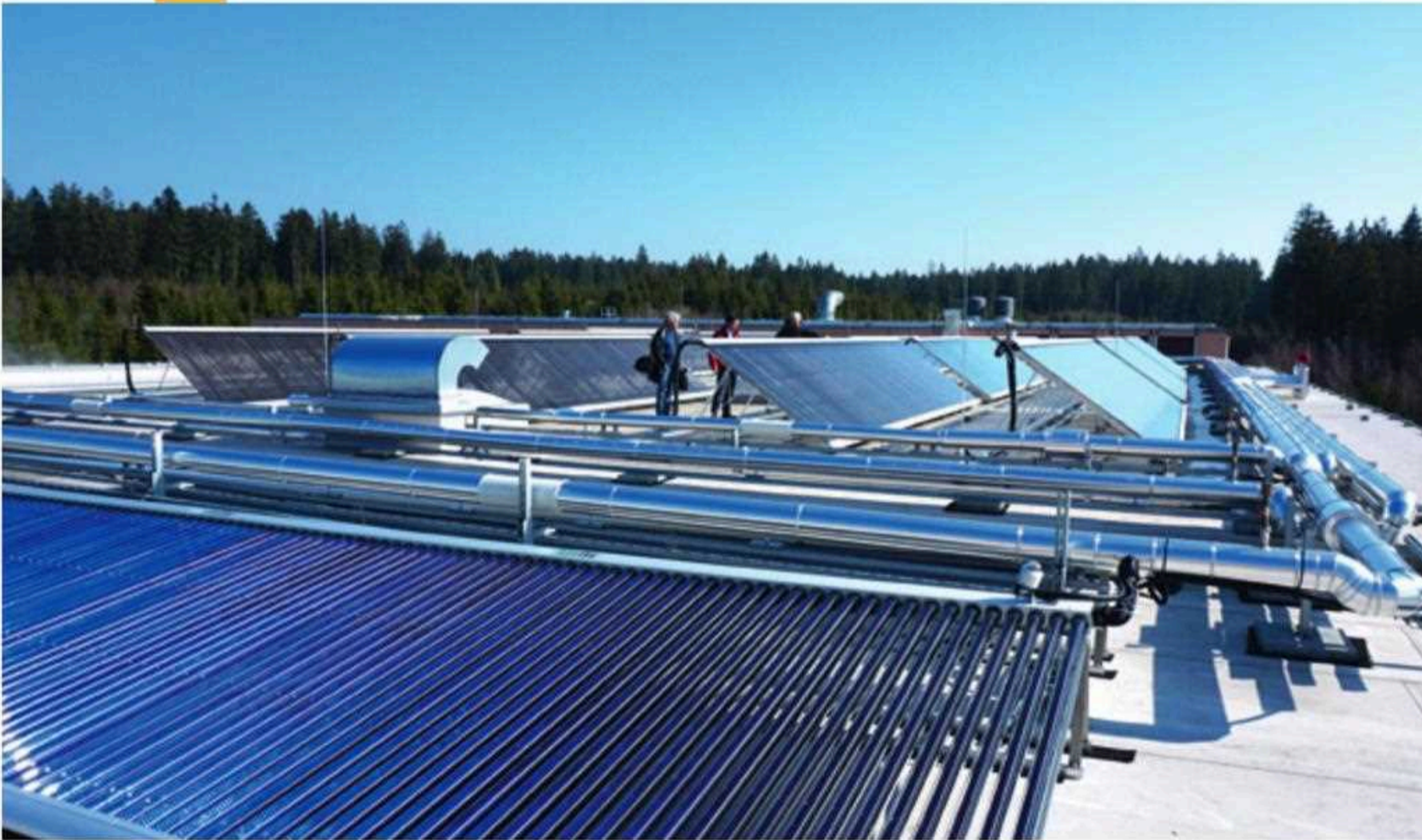
At the Rothaus brewery in Germany, almost 1,000 m 2 of vacuum tube collectors supply the bottle washing machines with heat Photo: Rothaus brewery, Germany
