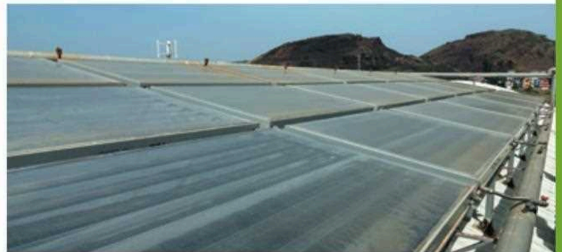
Heat from 294 m 2 of flat plate CPC (Compound Parabolic Collector) solar collectors drive a 70 kW water/LiBr absorption chiller for air-conditioning at the CERMI center in Praia, Cape Verde, since 2013 Photo: JER
