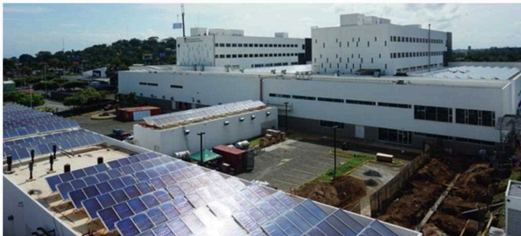
1 MW Solar cooling system at the Hospital Militar Escuela in Managua, Nicaragua Photo: SOLID Solar Energy Systems
