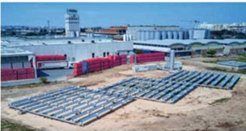
660 m 2 parabolic trough collectors for the Brewery Birra Peroni in Bari, Italy
