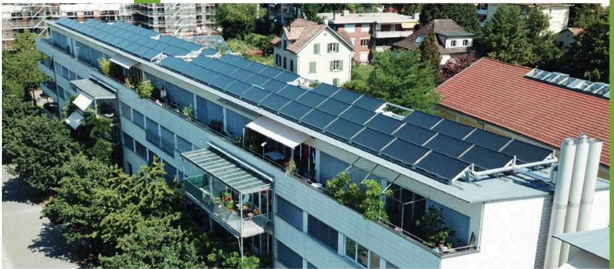
Multi-family house solar system “Im Werk” in Uster, Switzerland Photo: Soltop Energie AG, Switzerland
