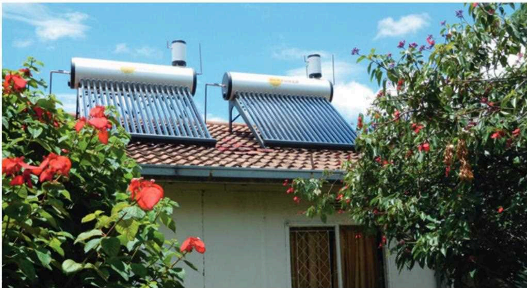
Thermosiphon systems at the CPS Sisters youth hostel in Harare, Zimbabwe Photo: Werner Weiss, AEE INTEC
