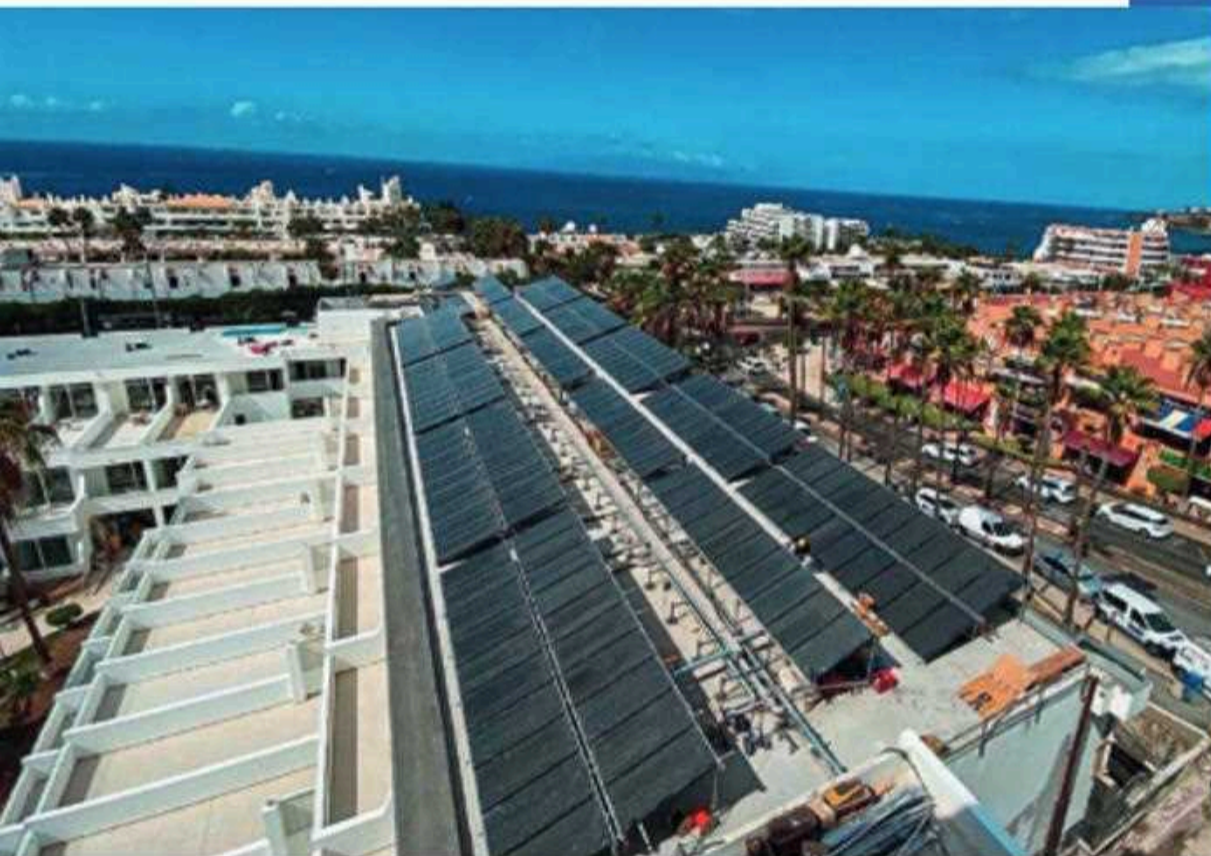
Photo: Abora Solar, Spain
