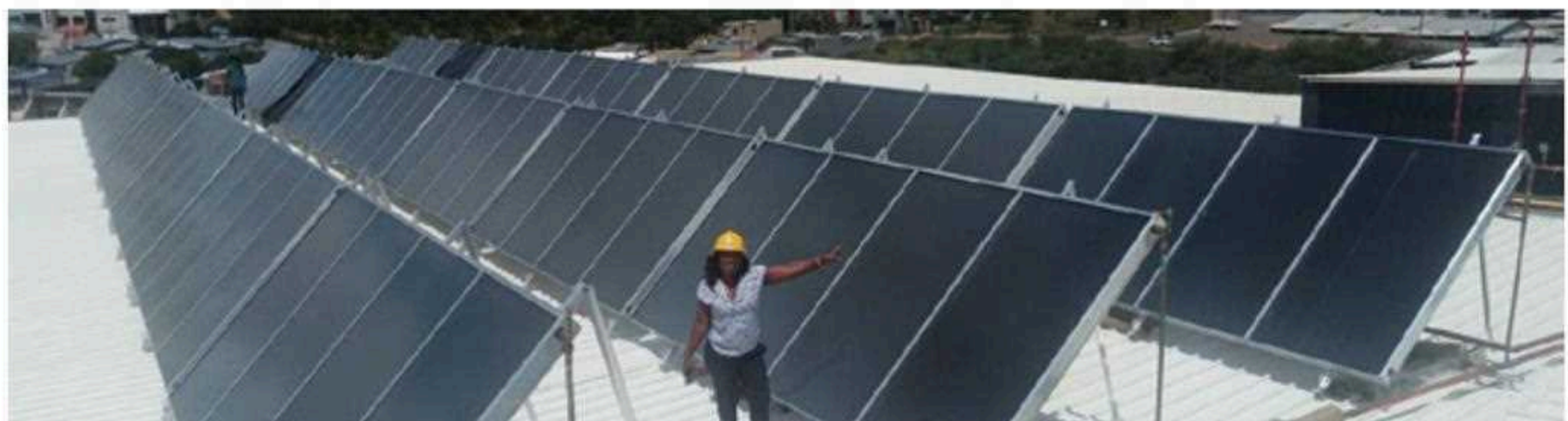
Pumped 210 m 2 flat-plate collector system at the Lady Pohamba hospital in Windhoek, Namibia Photo: Werner Weiss, AEE INTEC
