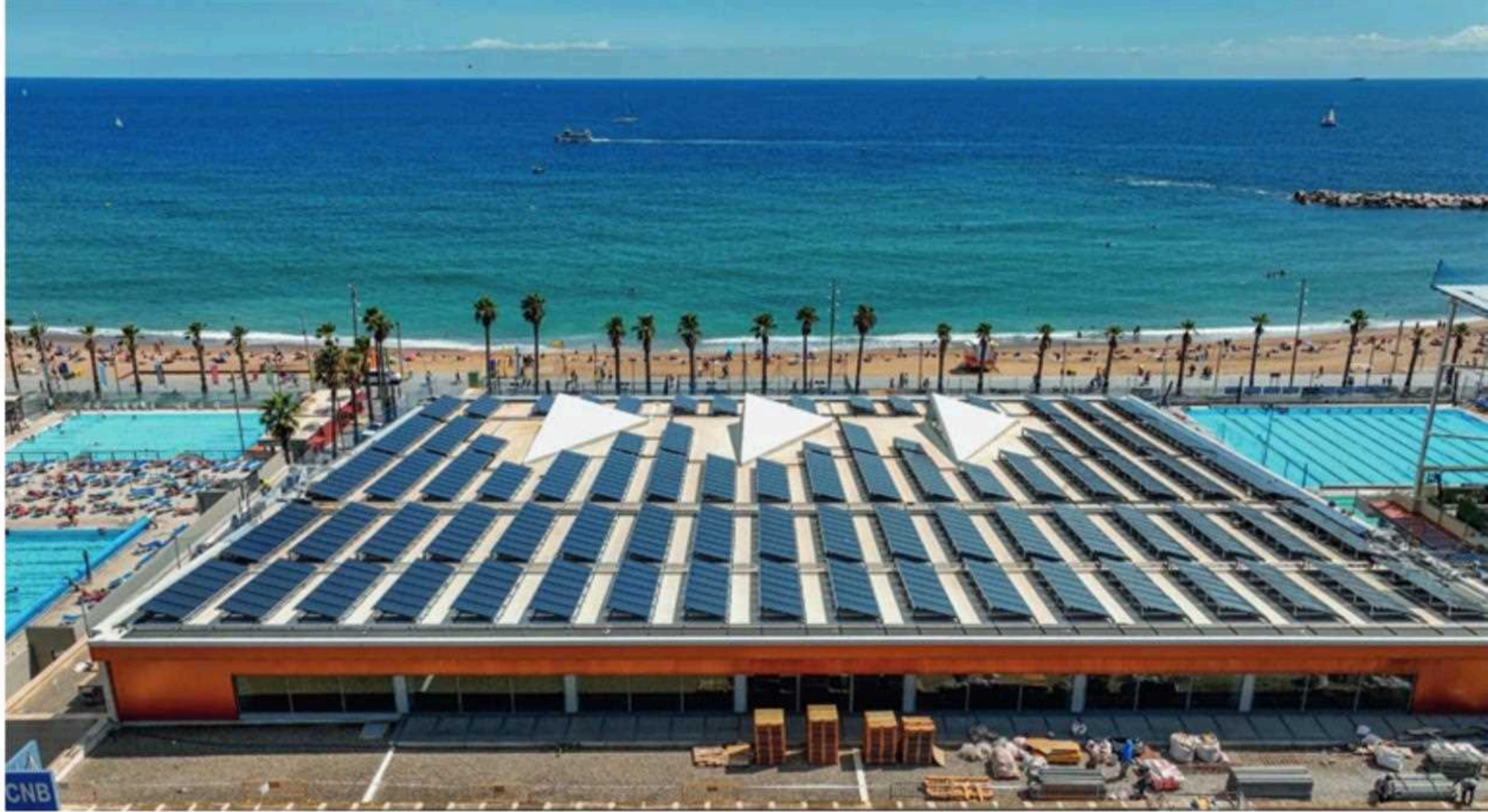
Domestic hot water and swimming pool system with 2,082 m 2 PVT in Barcelona, Spain Photo: Abora Solar, Spain
