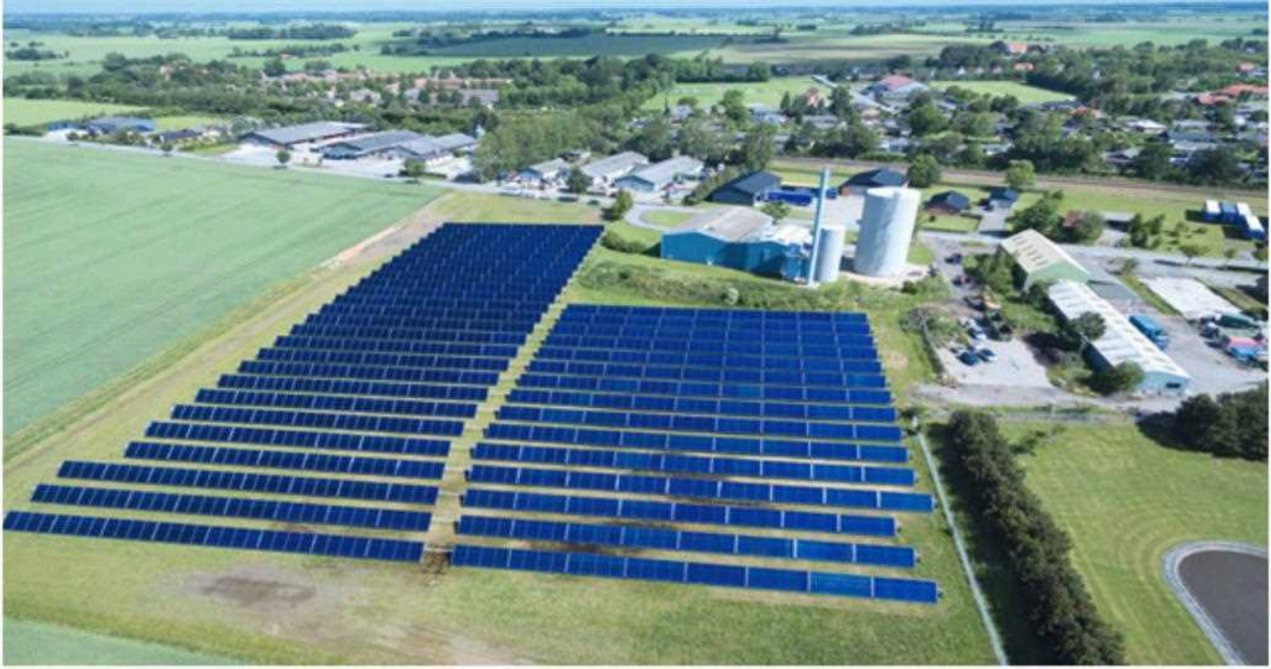
Solar district heating plant in Søllested, Denmark, consists of 4,700 m 2 double glazed flat plate collectors Photo: SavoSolar / Solar Heat Europe
