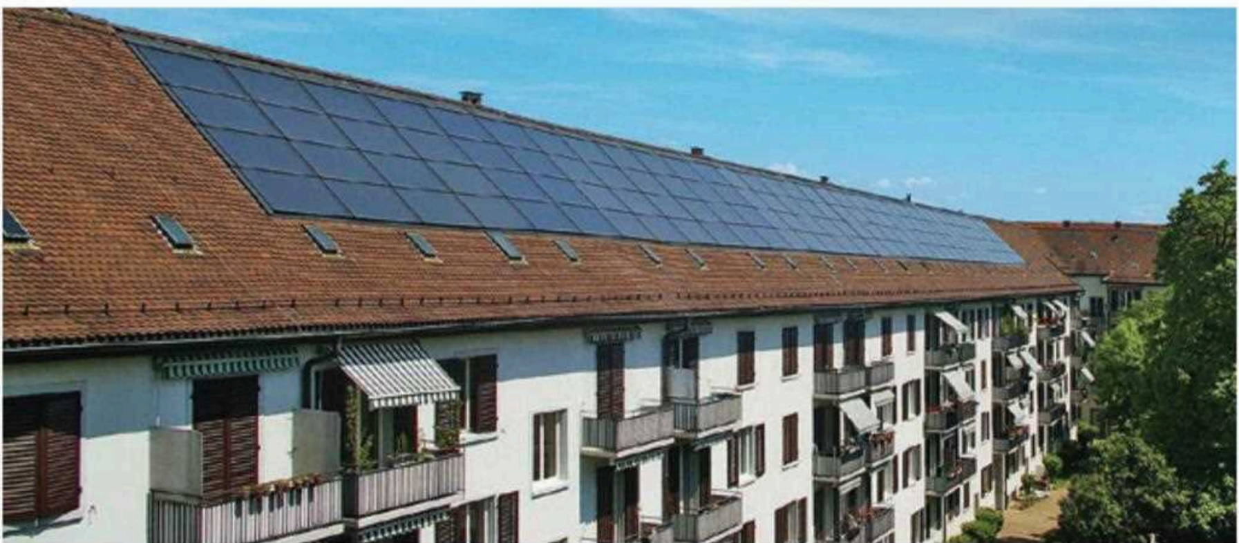
Solar thermal system for an apartment building in Zurich, Switzerland Photo: Soltop Energie AG, Switzerland
